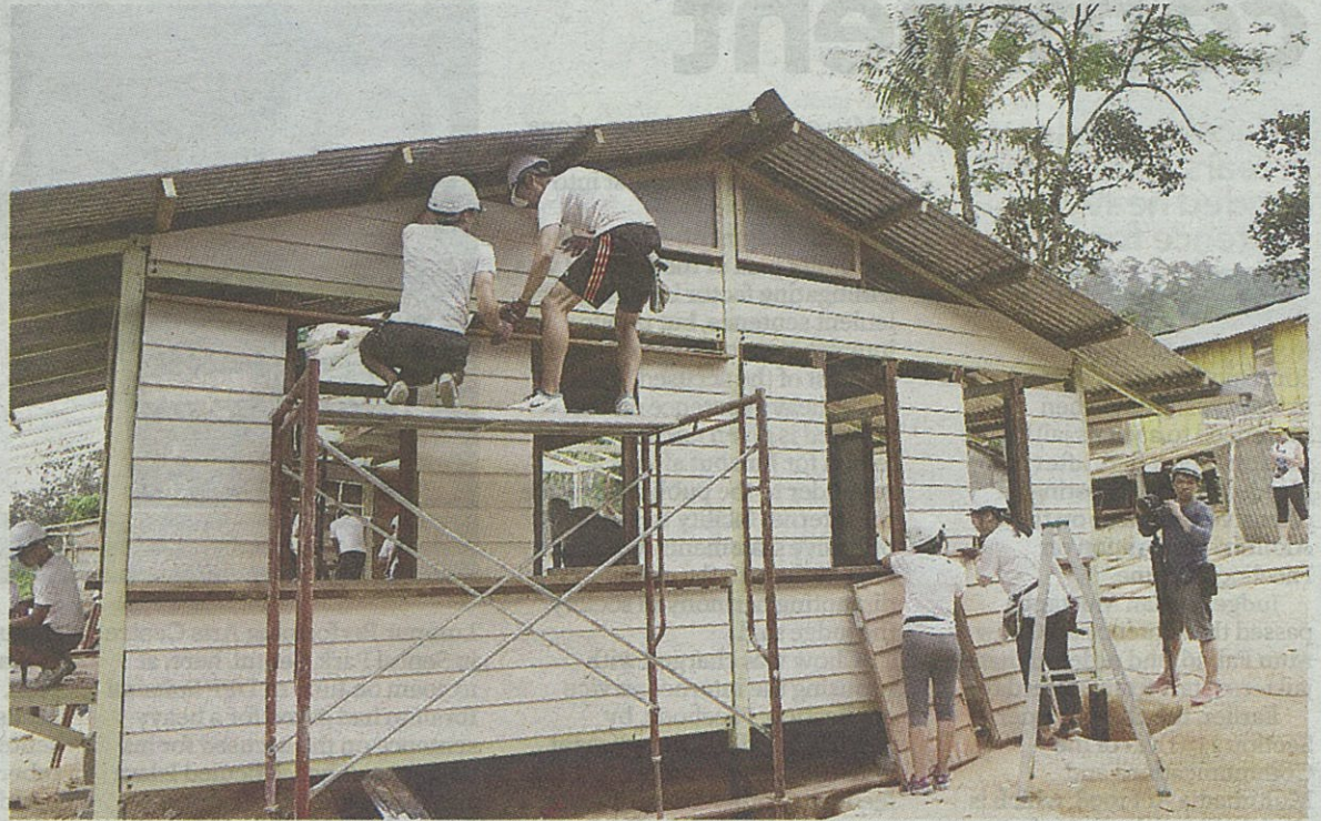
The house under construction by B.Youth volunteers for an orang asli family.
